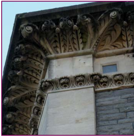
The deep eaves treatment on Pascoe House is embellished with an acanthus leaf motif.
